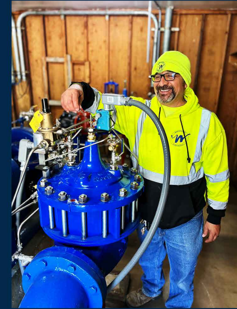
RENE MAGDALENO ELECTRICAL/MECHANICAL TECHNICIAN. 15 YEARS
